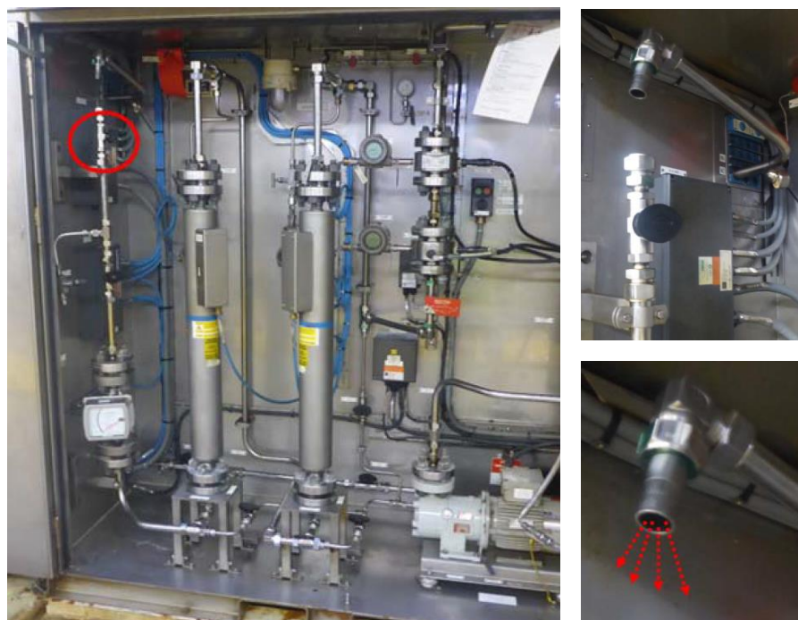
Figure: The red circle shows the site of diffuse leakage from the fittings on the analysis cabinet's final outlet valve. The 25mm tubing came loose when the operator tried to tighten the fittings. Oil and gas flowed out.
