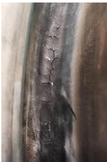
Figure 3: Perished and cracked air bellows.
