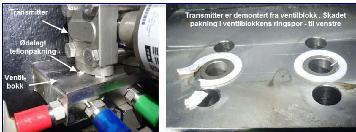
Figure: Destroyed teflon gasket between transmitter and valve block.
