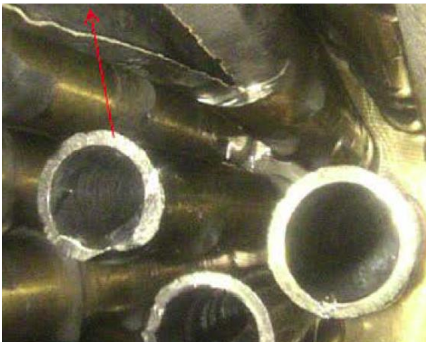
Figure 2: Video inspection after the incident. The leak site is marked with an arrow. Seen towards the cylinder plate.
