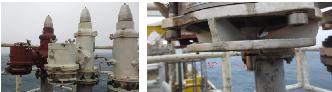
Figure 1 Left side: Pressure/vacuum valves (PVVs). Right side: Tap (full stroke check lift) considered to be modified.
