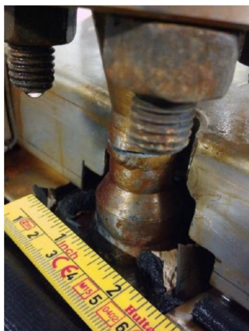
Figure 1 The leak point.
