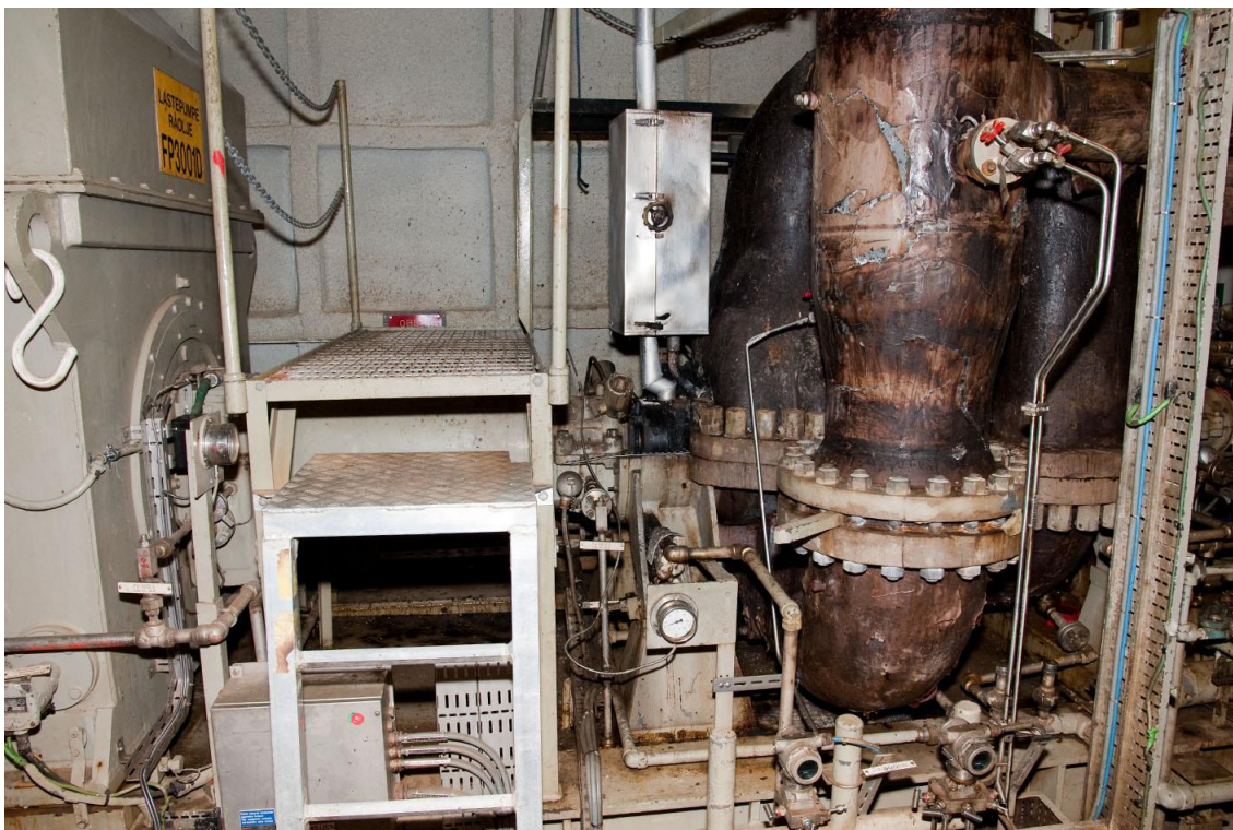
Photograph 4 - Fire damage at the drive end of loading pump D.
