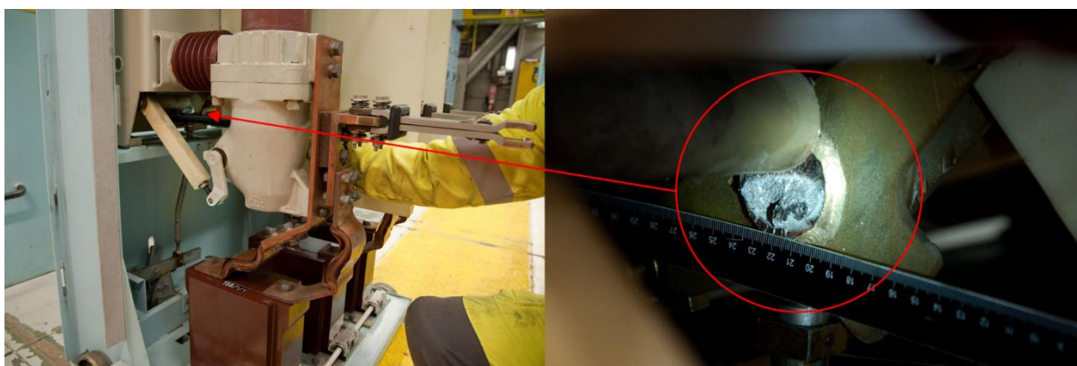
Photograph 2 - Fractured shaft in the circuit breaker for loading pump D.
