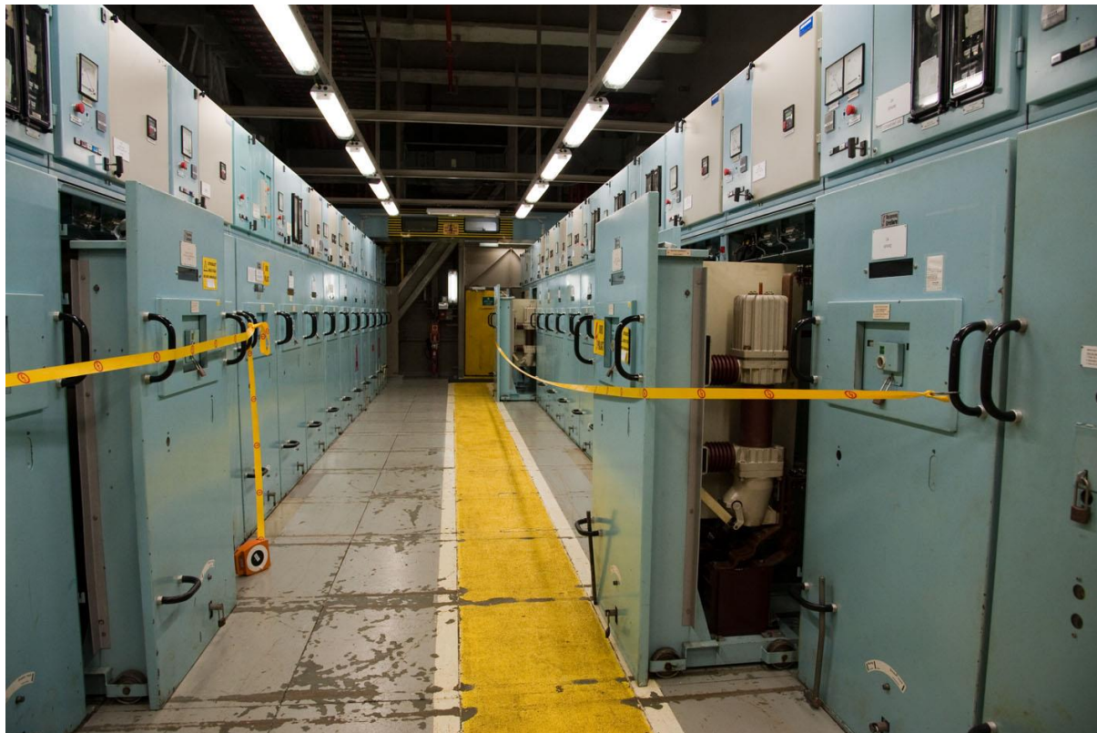
Photograph 1 - Circuit breakers in switchboard room KC0001.
