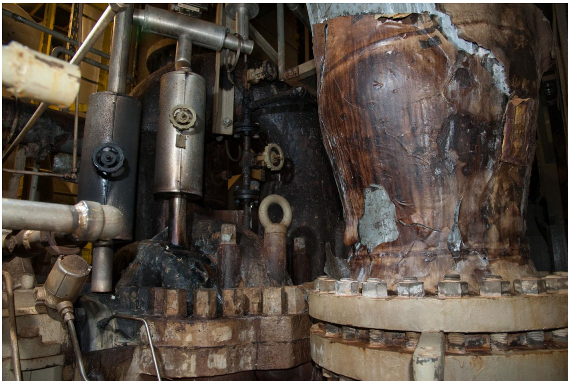
Photograph 5 - Fire damage at the free end of loading pump D.
