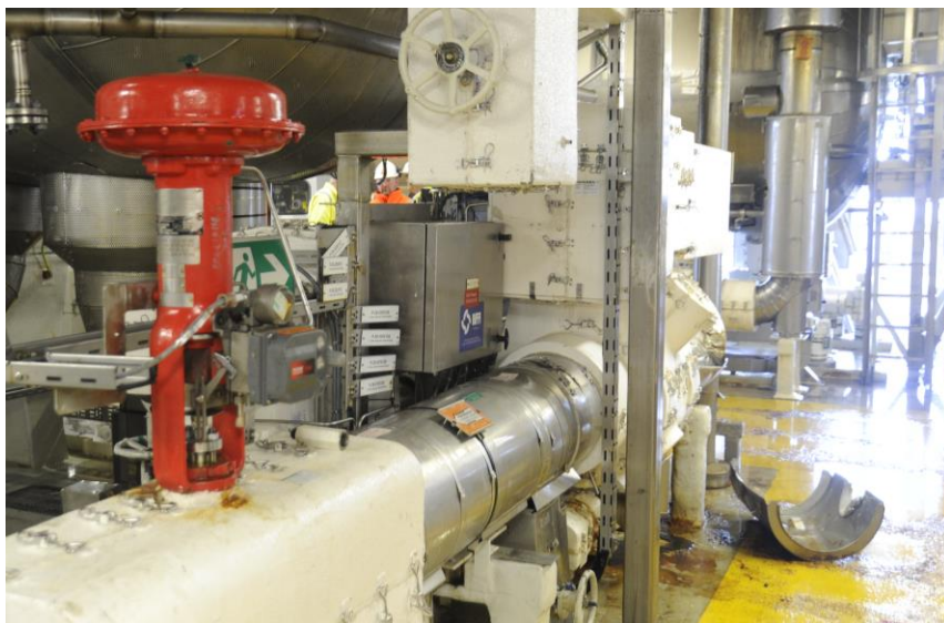
Figure 3: 20-LV0114 control valve (red). The cover below right was bent upwards by the leak and was removed to give access for sealing the leak site. (Photo: police)
