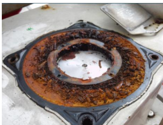
Figure 5- Opened actuator housing of the ESV, showing corrosion on the inside of the gasket. The photograph belongs to Engie E&P
