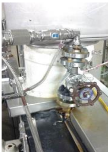
Figure 10 - Pipe nozzle and manual maintenance valve installed on condensate pump 23PA005B.
