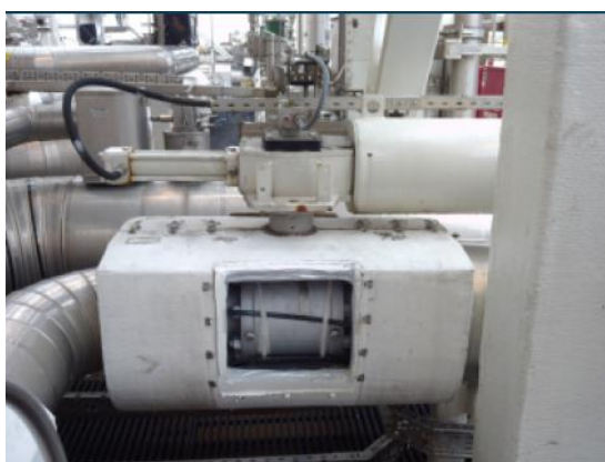
Figure 4- ESV with actuator installed. The photograph belongs to Engie E&P
