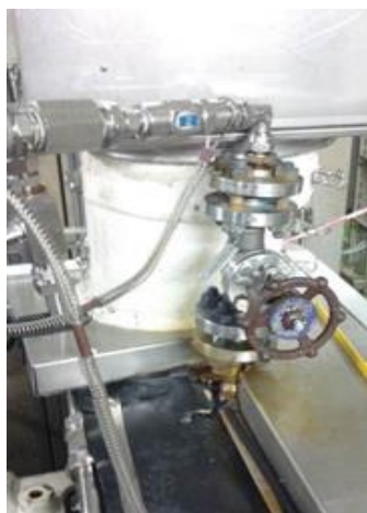
Figure 2 - Condensate pump with pipe nozzle. The photograph belongs to Engie E&P
