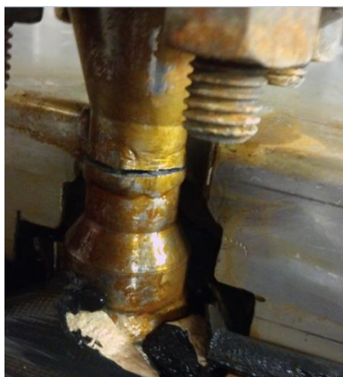
Figure 1 - Fracture in the pipe nozzle out of the condensate pump. The photograph belongs to Engie E&P
