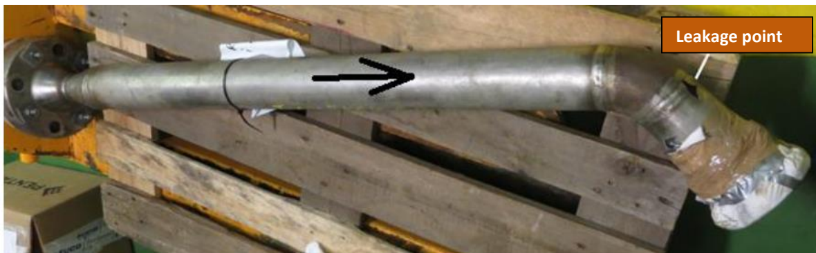
Figure: Depressurisation line with leakage. The arrow indicates the direction of the flow.
